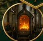
FORNO / CALDEIRA INDUSTRIAL
